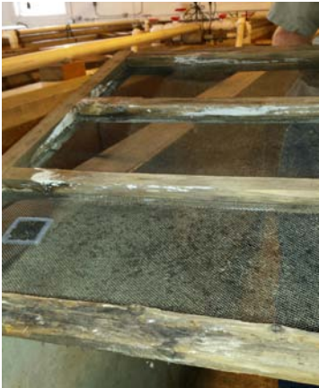
Figure 7: Rotting Fish Screen, one of several maintenance issues observed at ODFW hatcheries
